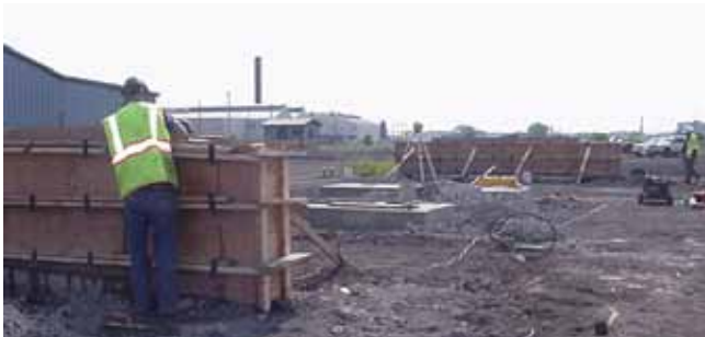
Figure 1 shows the work involved in preparing the site and foundation work to install the Heavy-Duty digital truck scale.
