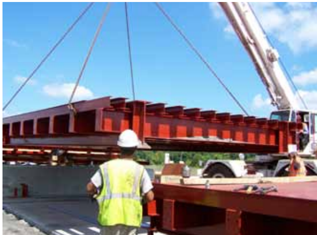
Figure 4 offers a view of the scale moved by crane, in line with the module already in place.
