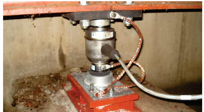
Figure 6 constraints of space for installation
