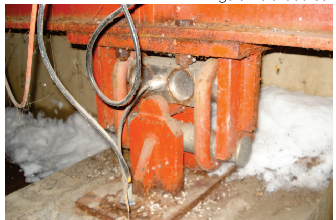
Figure 2 close up of old load cell
