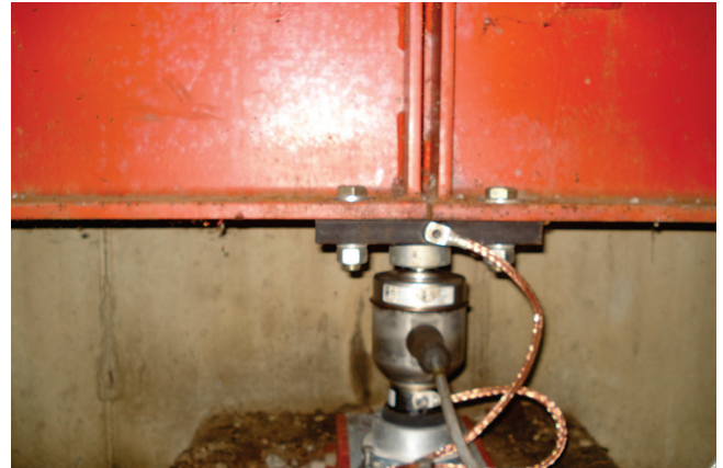
Figure 4 newly installed digital load cell
